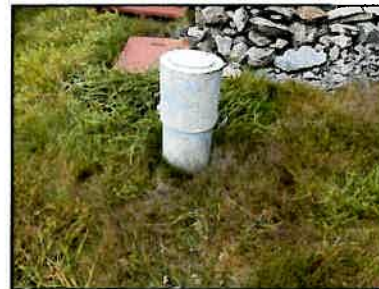
Sample of intact low voltage underground pillar
